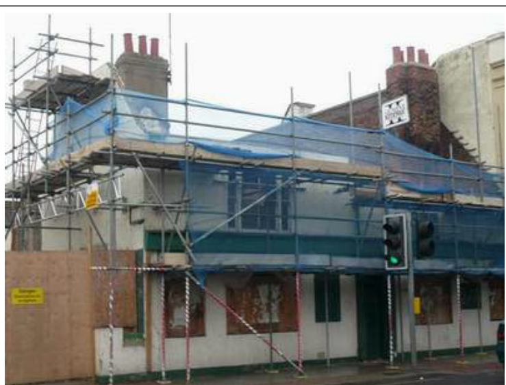
The former Guardsman Public House, in Fratton Road with its temporary roof covering.
